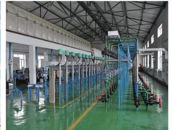
▲ 中国第一座三元复合驱配置注入站 China First Alkaline-Surfactant-Polymer (ASP) Flooding Injection Station
