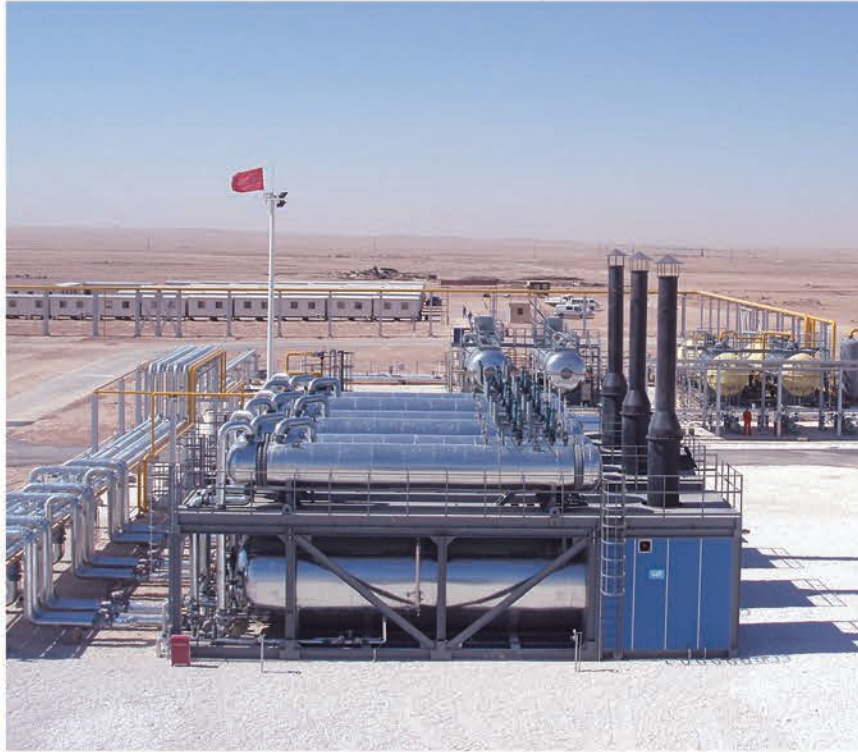
▼ 中东GBB油田CPF油气处理工程 GBB Oilfield CPF Oil & Gas Treatment Project in Middle East
