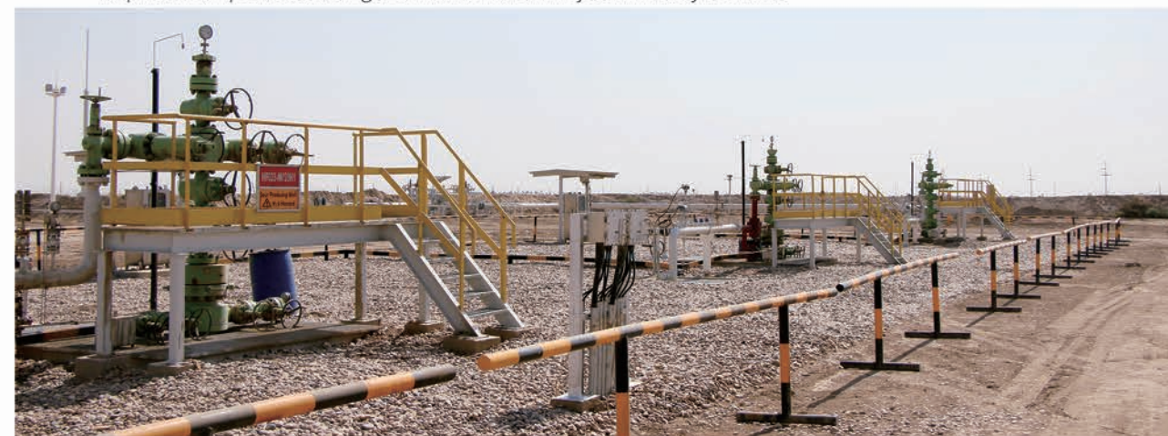
▼ 伊拉克哈法亚井间管线集输工程 Iraq Interwell Pipeline Gathering and Transmission Project in Halfaya Oilfield
