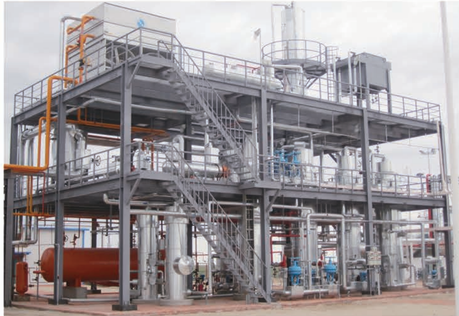
▼ 大庆呼伦贝尔油田注CO 2 提高采收率开发试验地面工程 Surface Engineering Project of Daqing Hulunbeier Oilfield CO 2 Injection to Enhance Oil Recovery
