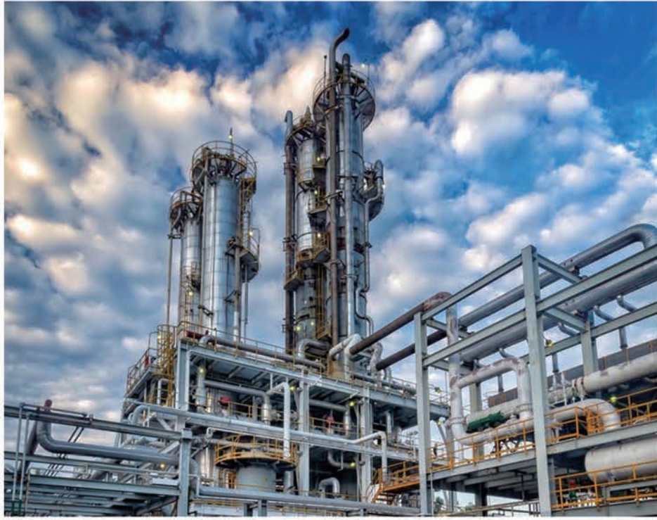
▼ 高尚堡油气处理厂天然气脱碳及CO 2 回收利用工程 Gaoshangbao Oil & Gas Treatment Plant Natural Gas Decarbonization and CO 2 Recovery Project
