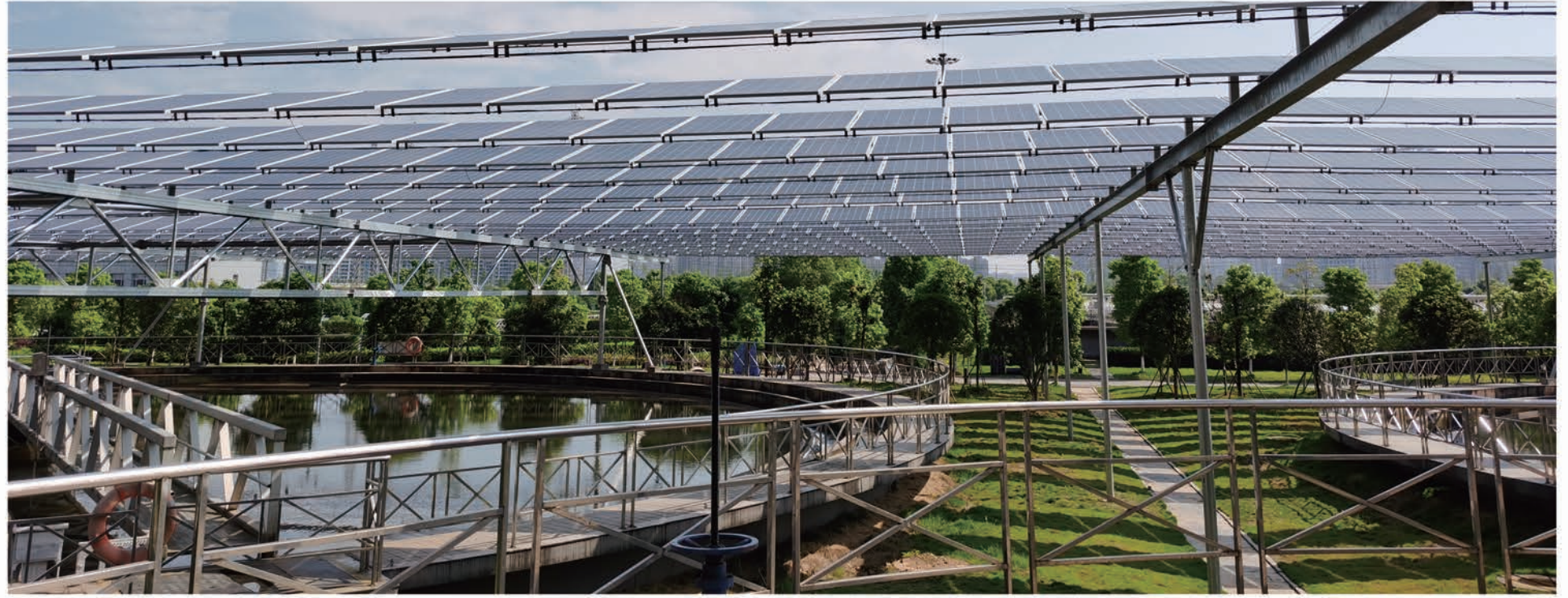
▼ 长沙水质净化厂分布式光伏工程 Distributed Photovoltaic Project of Changsha Water Purification Plant
