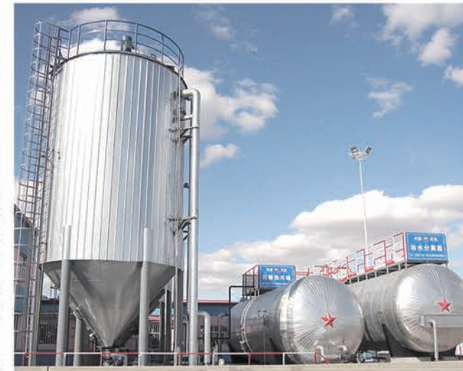
▲ 大庆油田采油一厂污泥处理现场 Daqing No.1 Oil Production Plant Sludge Treatment Site
