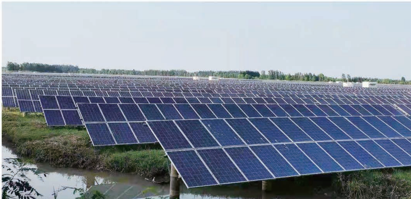
▲ 徐州亿通10MW渔光互补光伏工程 Xuzhou Yitong 10MW Fishing and Solar Complementary Photovoltaic Project
